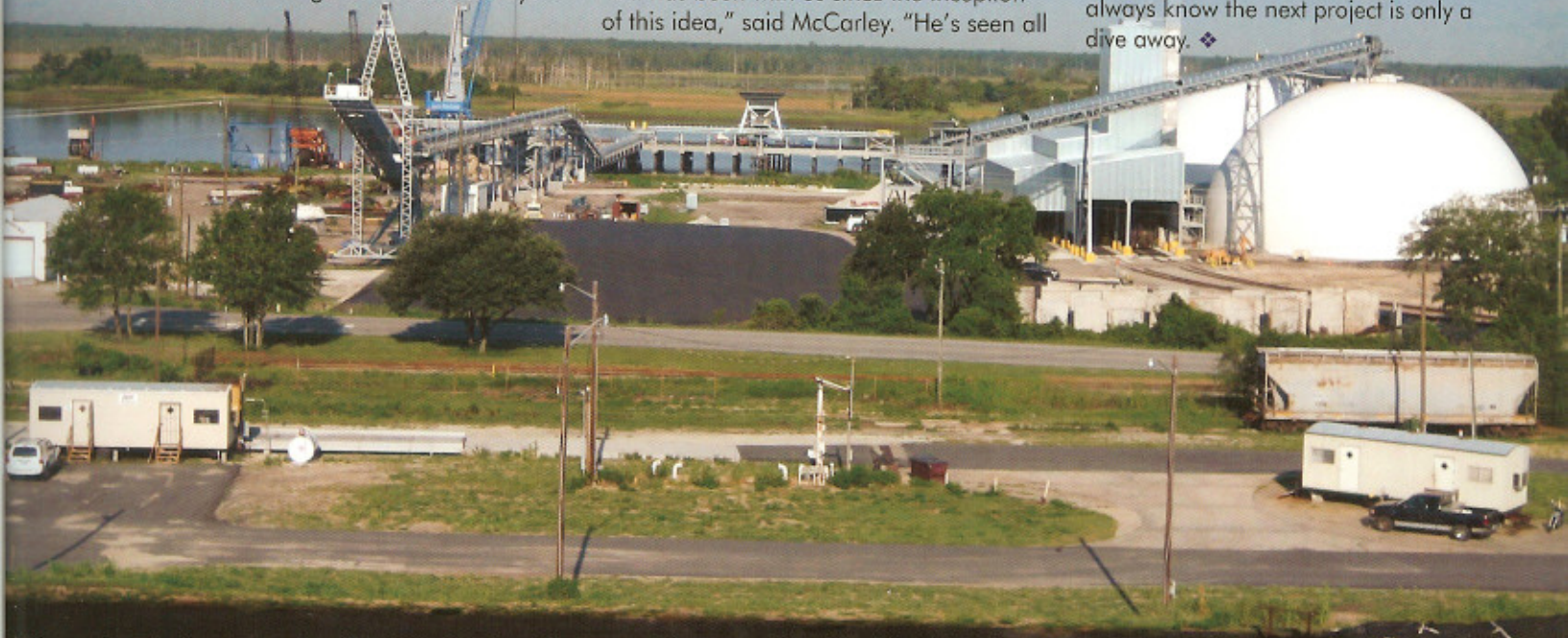
Shown here is the same site after construction. The expansion, completed in July 2006, features an enclosed conveyor system, two 15,000-ton concrete domes, and a high-speed rail and truck load-out system. Each of the domes is 70 feet high with a diameter of 140 feet. They are used to store urea, a chemical found in fertilizer. (Photo courtesy of Carolina Marine Terminal)
